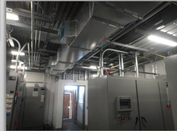
C88 Motor Control Room operating
