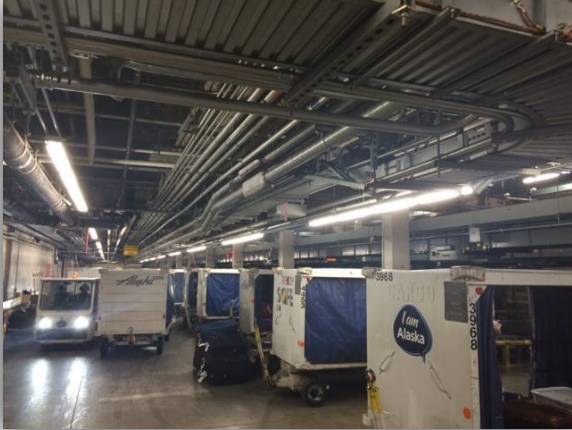
C88 Mainline 1 Conveyor back in operation
