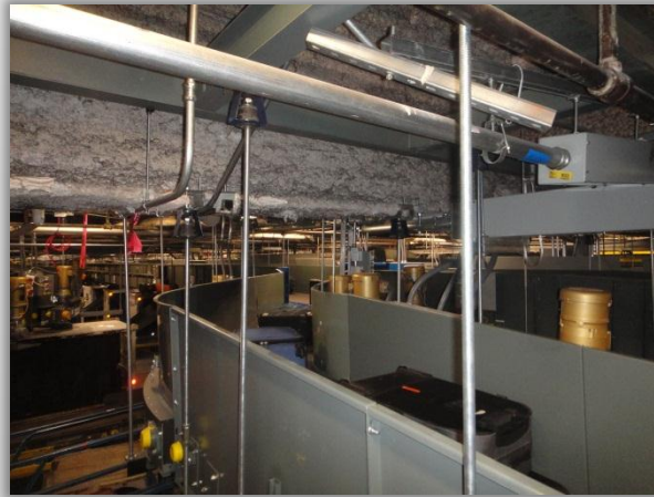
C88 Mainline 1 Operating
